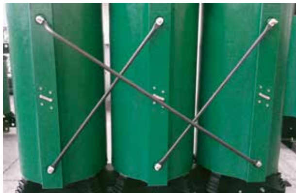
Example of HV terminals
