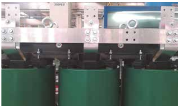
Example of LV terminals
